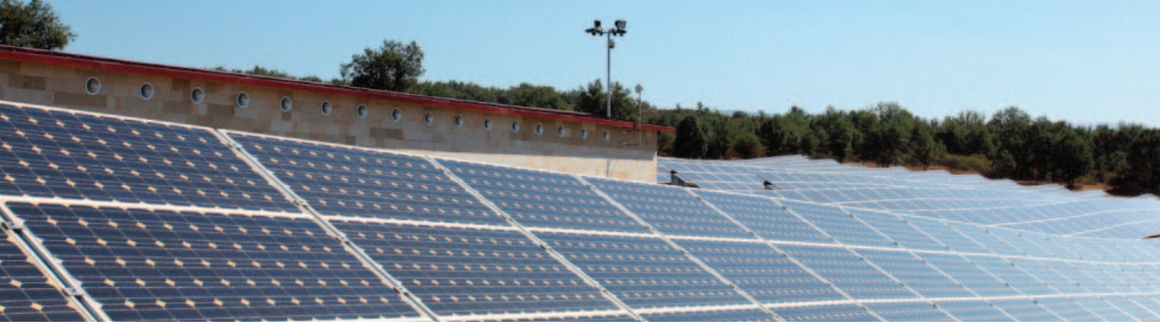
Element Power owned Las Pinares Solar Facility, Spain
