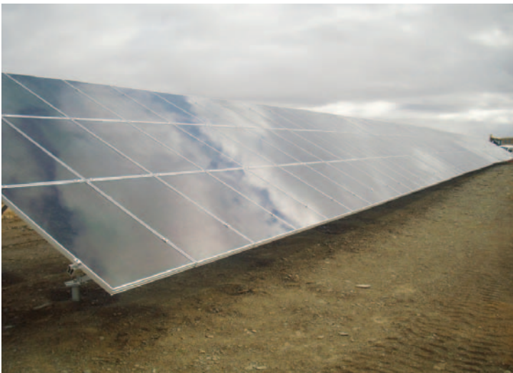
Element Power-owned Pascuales Solar Facility, Spain
