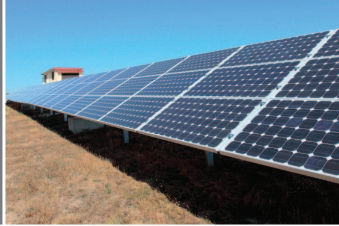
Element Power owned Las Pinares Solar Facility, Spain
